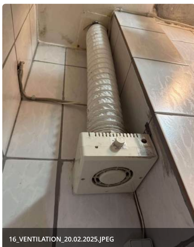
Ventilation i bad
