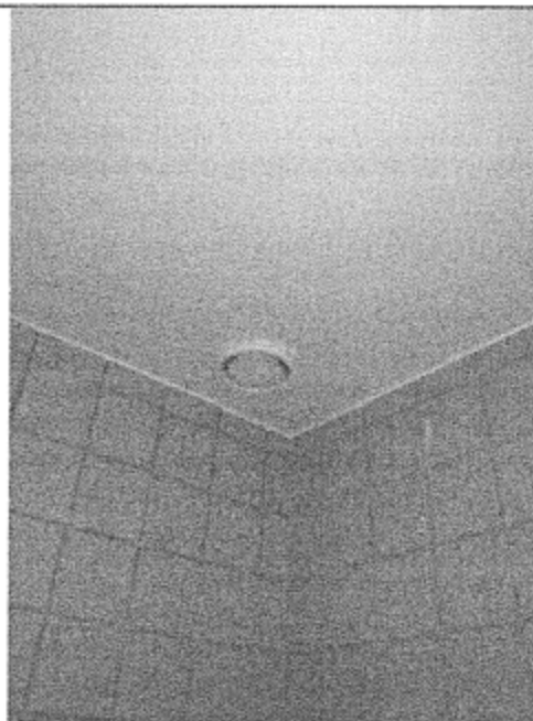
Ventilation i bad
